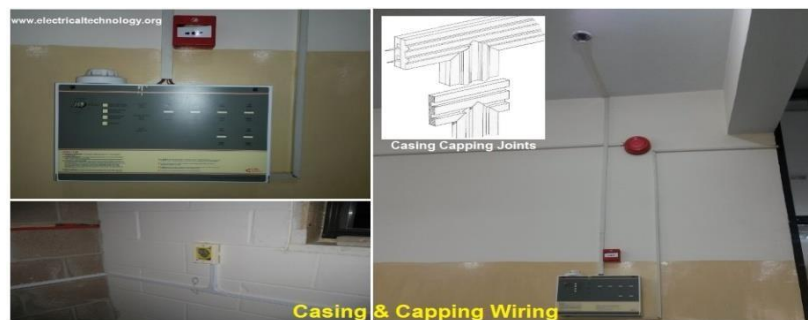
Fig.2.5. Wooden casing and capping wiring.
