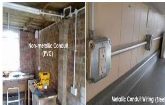
Fig.2.8. Surface conduit wiring.
