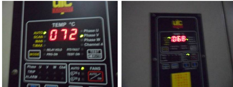
Figure1--: Temperature reading of transformer in power distribution room 1112
