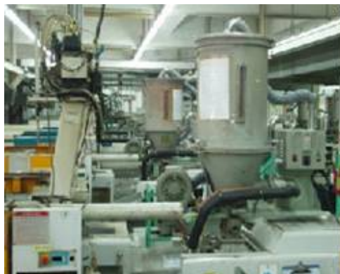
Figure 5-4: Heat recycling equipment for an injection-molding machine
