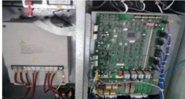
Figure 2-7: Elevator network controller
