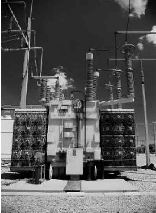
FIGURE 4.16 A large power transformer. Source: http://images.google.com/images?q=photos+of+power+transformers
