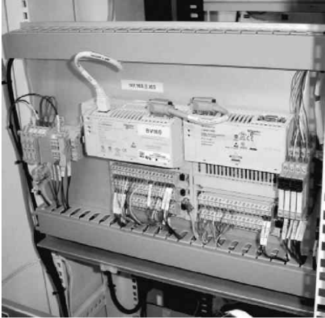
FIGURE 8.2 Example PLC installation.
