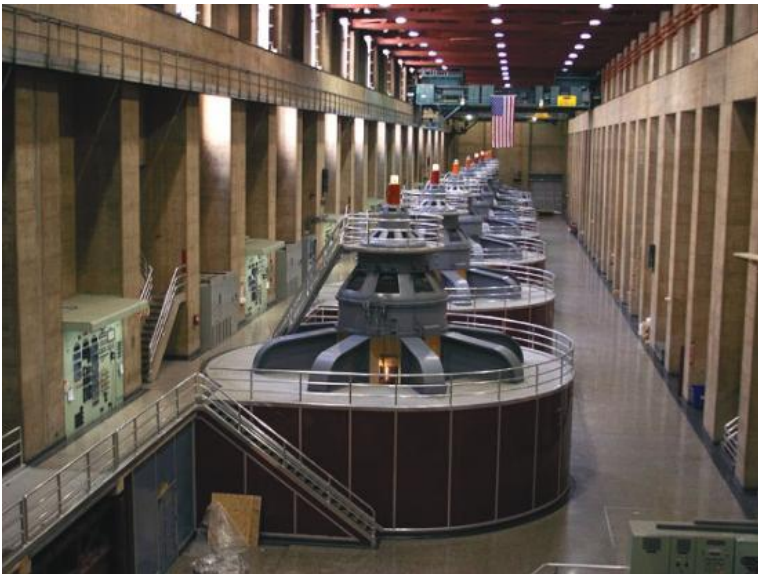
(b) Generating Hall: Hoover Dam
